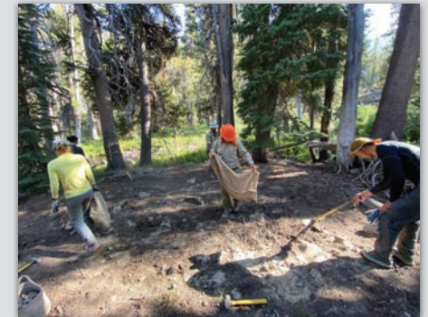
Restoration crews working on a highly-impacted site along the Shadow Creek corridor.
